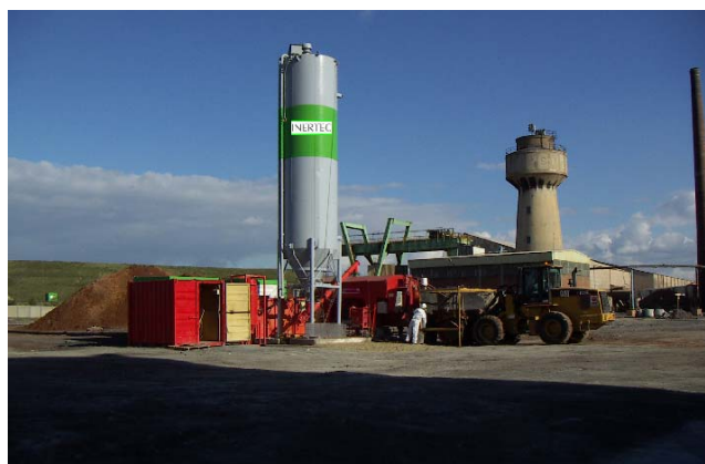
Mobile residue treatment unit
